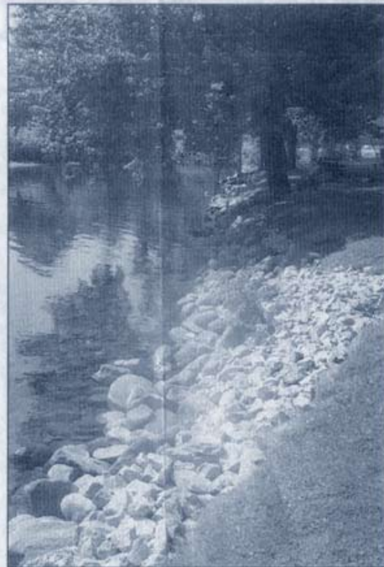
One of the biggest washed-out areas at Norcross Point was filled in fully with new granite stones. Other stones were retrieved from the water.
